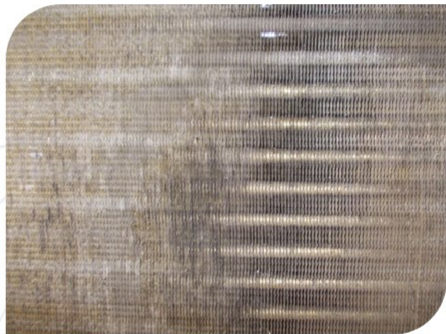
GAS COOLER BEFORE COATING
